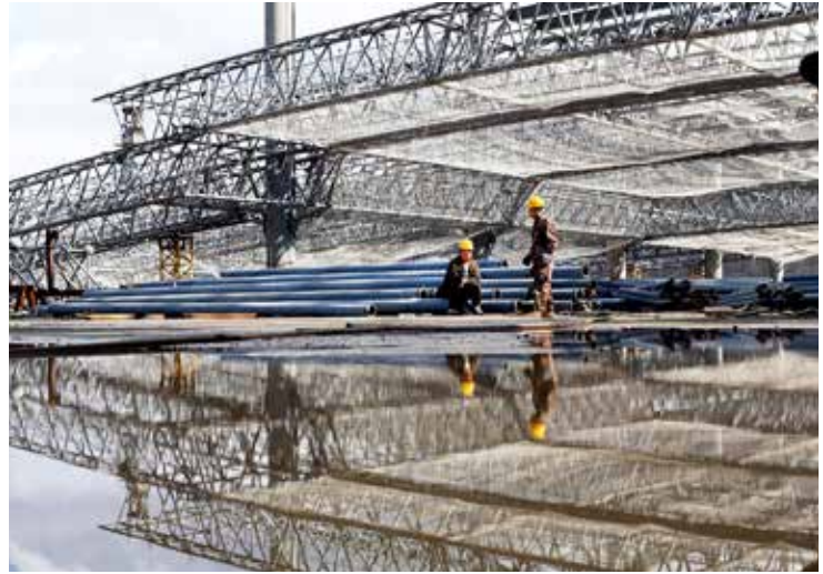
November 3, 2015: Kunming South Railway Station under construction in Kunming, capital of Yunnan Province. Four major rail links, including the Lanzhou-Chengdu-Kunming Line, the Shanghai-Kunming Line, and lines running to coastal areas of southern China and to southwestern China, as well as the Pan-Asia Rail Network, converge at the station. [CFP]
